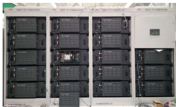
图 13 BSR21-01-C 储能电池架 Fig. 13 Energy storage battery rack of BSR21-01-C
