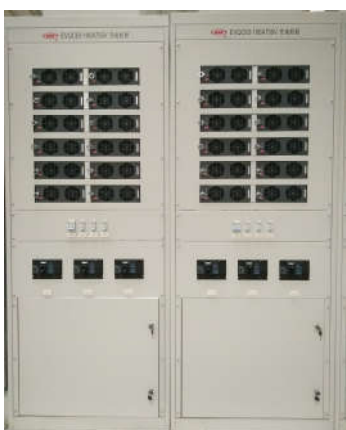
图 10 EVQC63-180A750V 充电机柜 Fig. 10 Charging cabinet of EVQC63-180A750V
